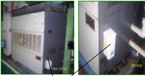
Intelligent controllers installed on site
