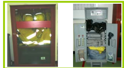
Fire Combats Equipment
