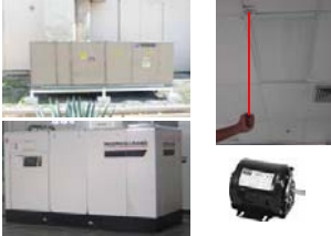
Stop equipments, A/C , Exhaust motor fans, production equipment, air compressor,
